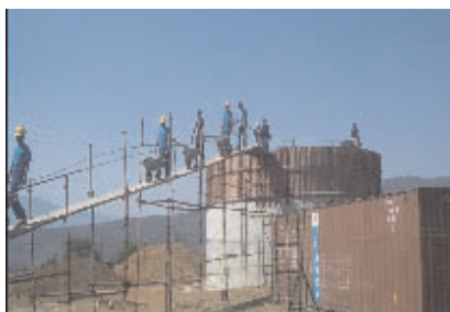
Ndaya Water Supply
